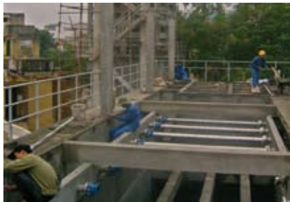
2H TUBEdek® Kim Lien potable water plant in the centre of Hanoi: Lamella clarifier equipped with TUBEdek®
